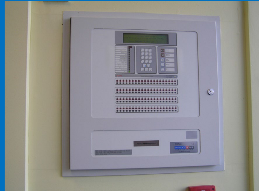
Addressable Fire Alarm Panel
