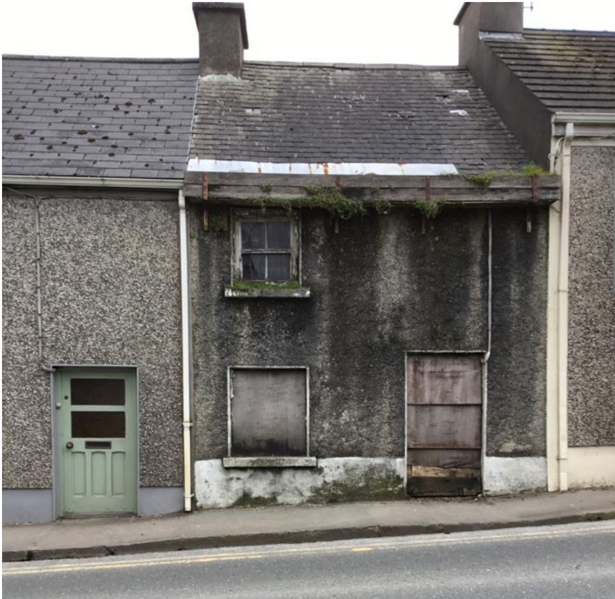
Figure 6-9: Derelict Residential Building on Limerick Street.
