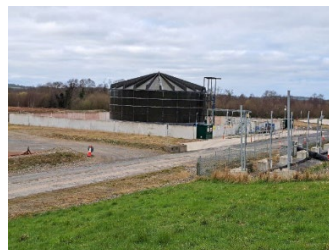
Ballaghveny Landfill – Leachate Storage Area
