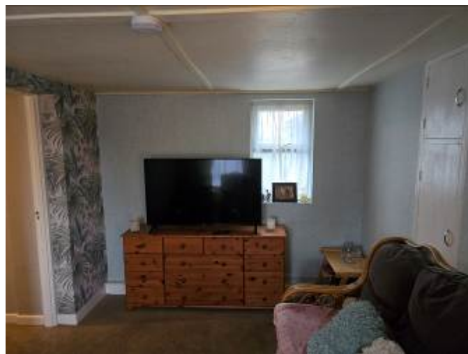
17. Window ope altered to form new Back Door. Soft Board Ceiling to be replaced.
