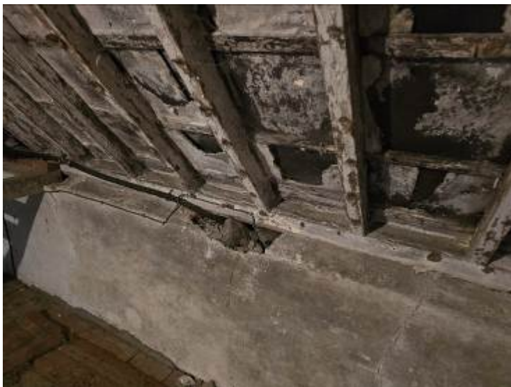
18. 19. 20. 21. Attic overhead. Lime parging to be removed as part of Re Slating.
