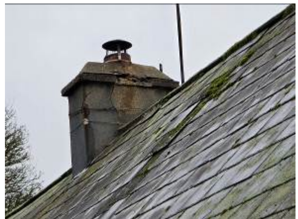
11. Chimnery to be Re Capped and RE Plastered Roof to be Re Slated
