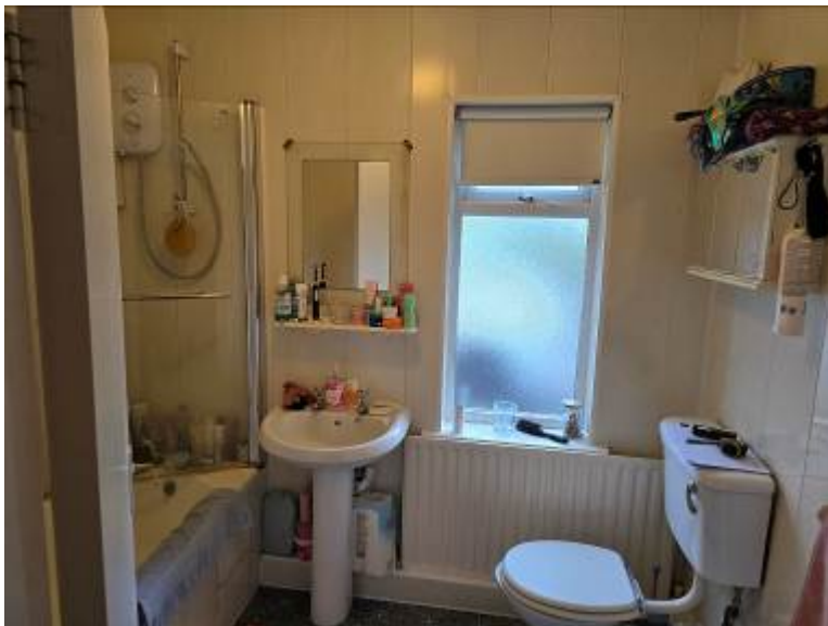
25. Bathroom Suite to be replaced.
